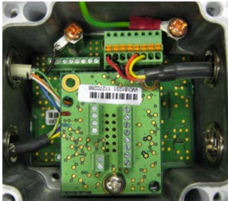
Figure 4 Hub Box with Digital Pec fitted.
