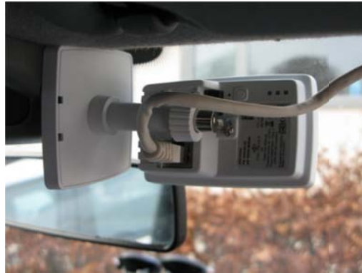
Overhead camera mounted – seen from the inside
